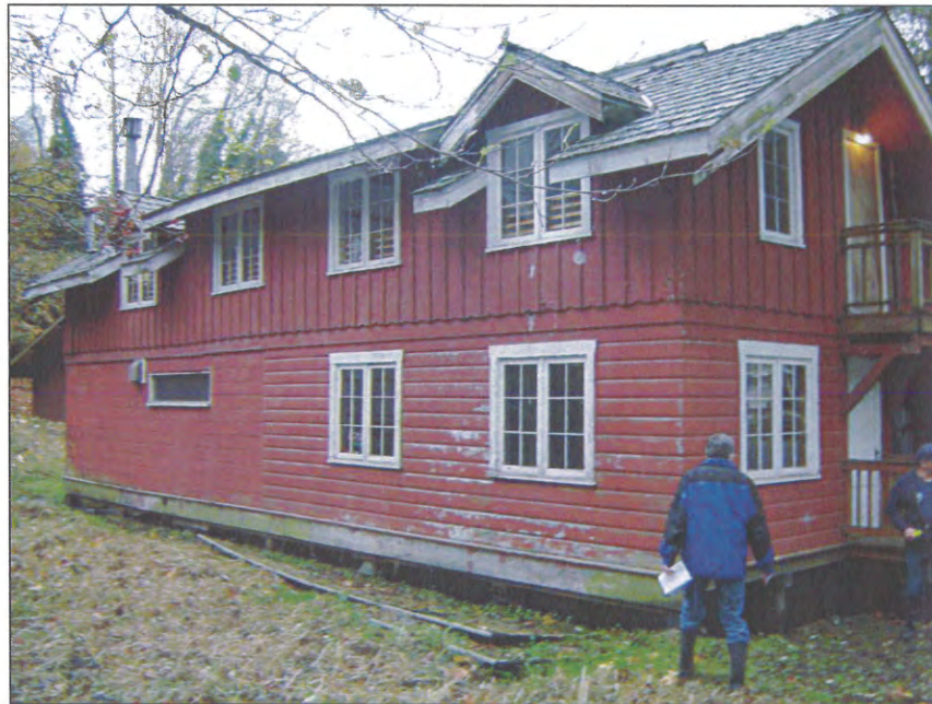
West and partial north facades of the Sun Home Lodge. Note proximity of the wood to grade, and the deteriorated paint.
