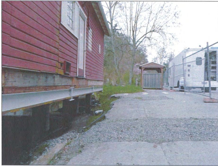
East side of the Dining Hall looking north. Note the damaged service drive paving, Deteriorated retaining wall (left) and bus stop (center).
