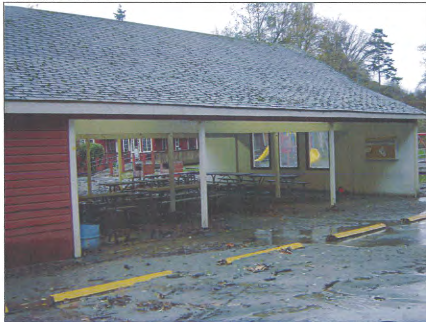
Picnic Shelter looking southeast from the parking lot, with sediment and site drainage running through the building.
