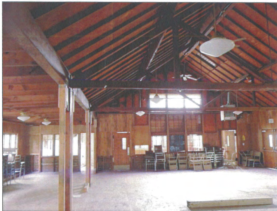
Interior of the Dining Room, looking south. Note exposed roof structure, posts, and sediment-laden decorative plywood floor.
