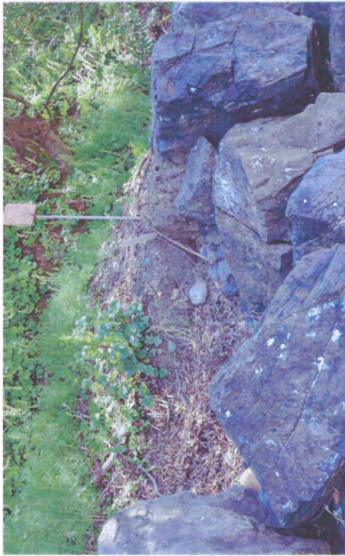
Toppled Bulkhead Area Needing Repair
