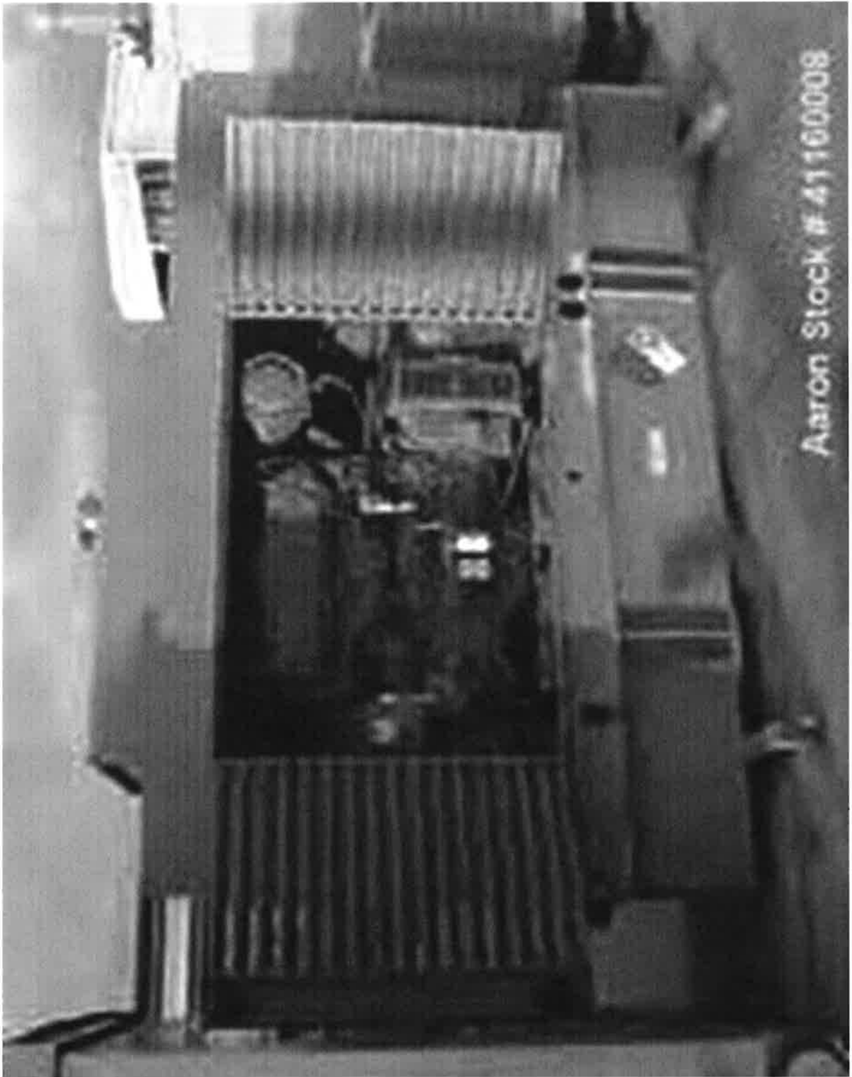
City Hall Generator
