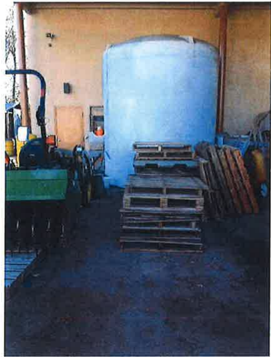
06 DESCRIPTION: DE-ICER TANK UNDER COVER WITHOUT SECONDARY CONTAINMENT.
