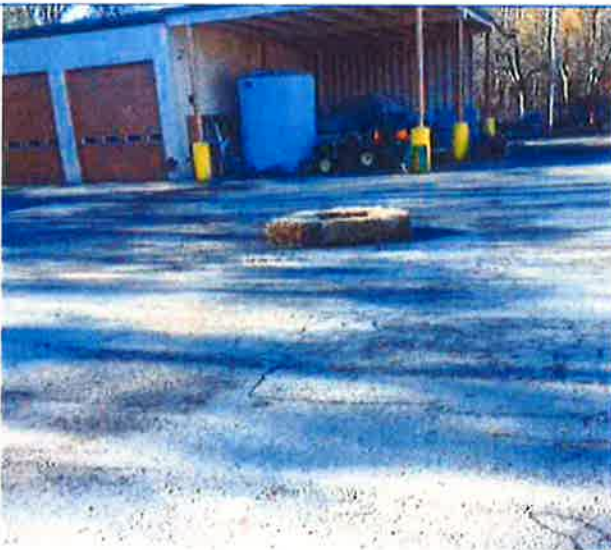
(BEFORE) Photo 10: HAY BALE BERM SURROUNDING CATCH BASIN IN VEHICLE WASH AREA.
