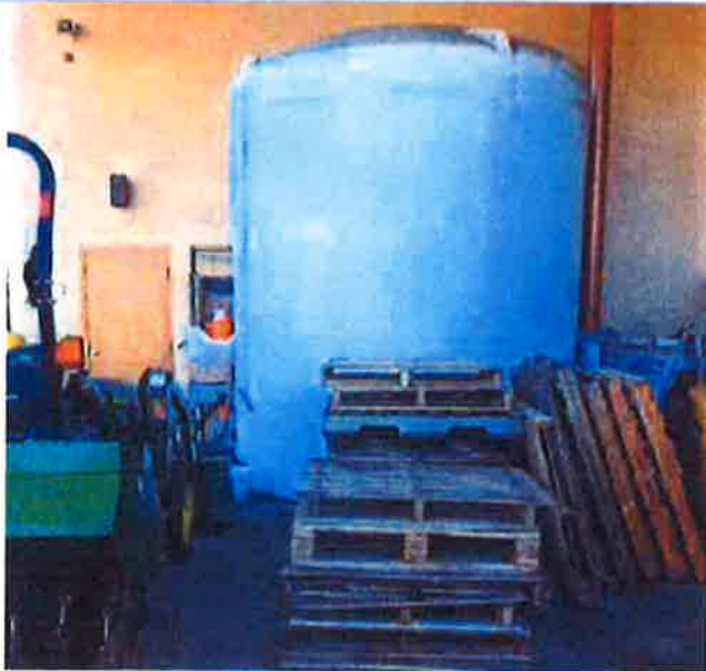
(BEFORE) Photo 06: DE-ICER TANK UNDER COVER WITHOUT SECONDARY CONTAINMENT.
