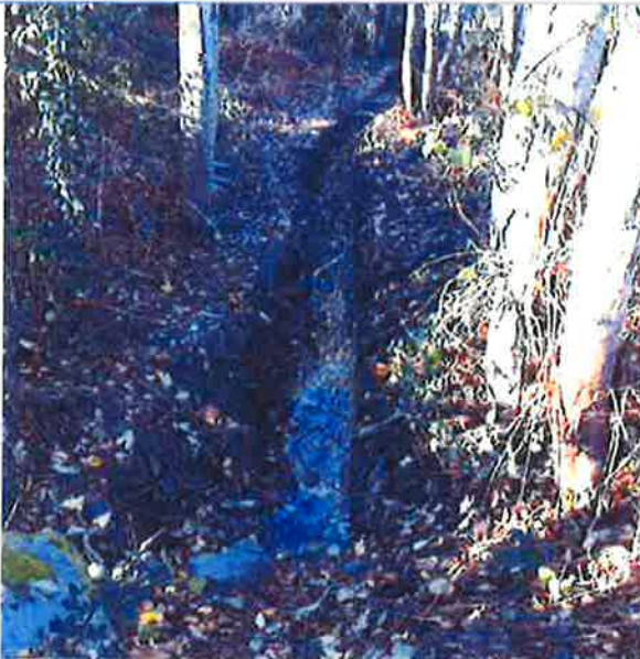
(BEFORE) Photo 16: RECENTLY EXCAVATED UNSTABILIZED DITCHLINE FROM WESTERN STORMWATER CONVEYANCE AND DETENTION PIPE TERMINUS TO STREET DITCHLINE. TERMINUS OF ON-SITE STORMWATER SYSTEM AT BOTTOM OF PHOTO.
