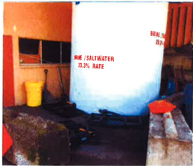
(AFTER) Photo 06-A: DE-ICER TANK IS STILL NEEDED SECONDARY CONTAINMENT. THE TANK HAS BEEN LABELED AND A SPILL KIT WITH DRIP PANS HAVE BEEN ADDED TO THE AREA.
