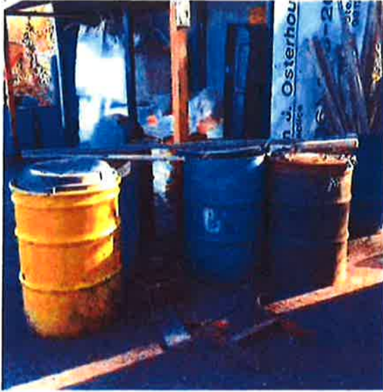
(BEFORE) Photo 07: SOUTH FENCELINE MATERIAL STORAGE. POLLUTION GENERATING MATERIAL EXPOSED TO RAINFALL. SAND BAGS UNDER COVER TO PREVENT DETERIORATION.
