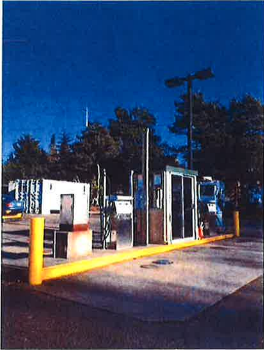
13 DESCRIPTION: FUELING ISLAND
