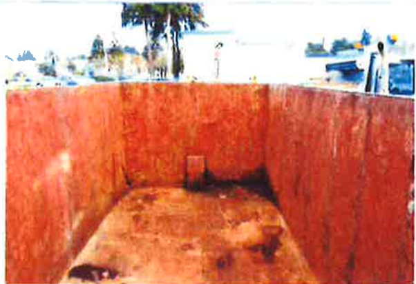
(AFTER) Photo 03-A: SCRAP HAS BEEN EMPTYIED. REPLACEDMENT BIN HAS BEEN ORDERED WITH COVER.
