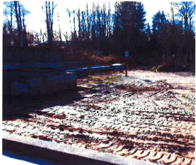
(AFTER) Photo 15-A: MAJORITY OF POLLUTION GENERATING MATERIAL HAS BEEN RELOCATED UNDER COVER OR DISPOSED OF PROPERLY.
