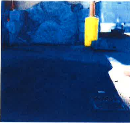
(BEFORE) Photo 05: COVERED SALT PILE IN CLOSE PROXIMITY TO CATCH BASIN.
