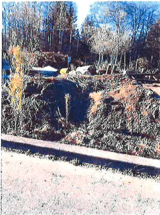
15 DESCRIPTION: MATERIAL STORAGE (SOIL, METAL, CONSTRUCTION DEBRIS) OUTSIDE FENCE (NW CORNER). POLLUTION GENERATING MATERIAL EXPOSED TO RAINFALL.
