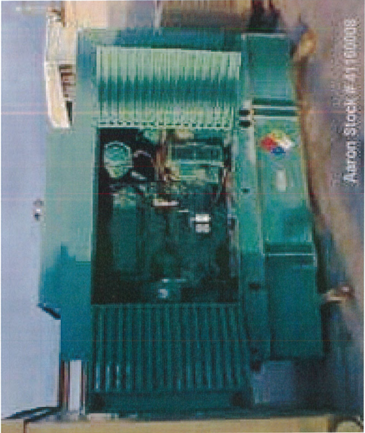
City Hall Generator
