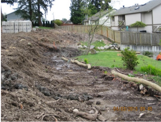
Photo 5. Construction Site Needing Enforcement Measures.
