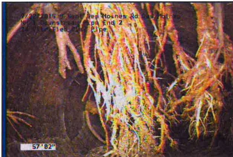
Photo: NA_MH 1_Pipe End 2_S Kent Des Moines Rd_22092015_131651_A.JPG, VCR No.: 9.22.2015 50.2FT, Roots Tap Joint, from 10 to 02 o'clock, 20 %, within 8 inches of joint: YESR, Start
