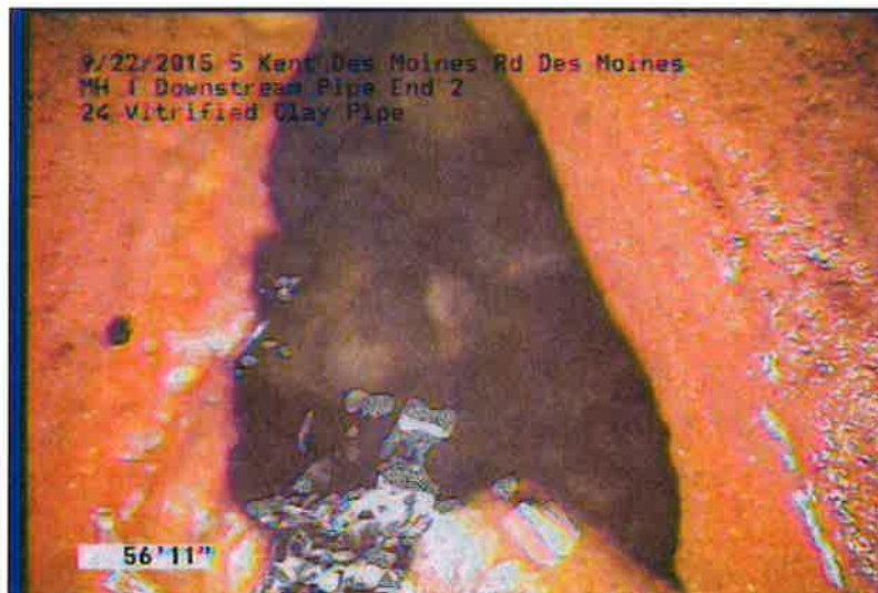
Photo: NA_MH 1_Pipe End 2_S Kent Des Moines Rd_22092015_145507_A.JPG, VCR No.: 9.22.2015 56.95FT, Hole Soil Visible, from 05 to 06 o'clock, within 8 inches of joint: YES
