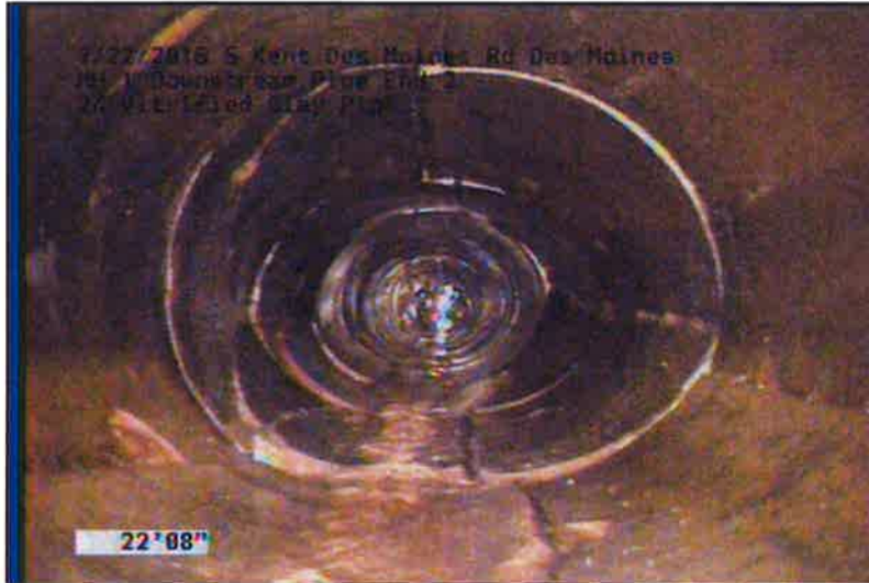
Photo: NA_MH 1_Pipe End 2_S Kent Des Moines Rd_22092015_145203_A.JPG, VCR No.: 9.22.2015 20.4FT, Fracture Longitudinal Hinge, 4, from 12 to 12 o'clock, within 8 inches of joint: YES, Start
