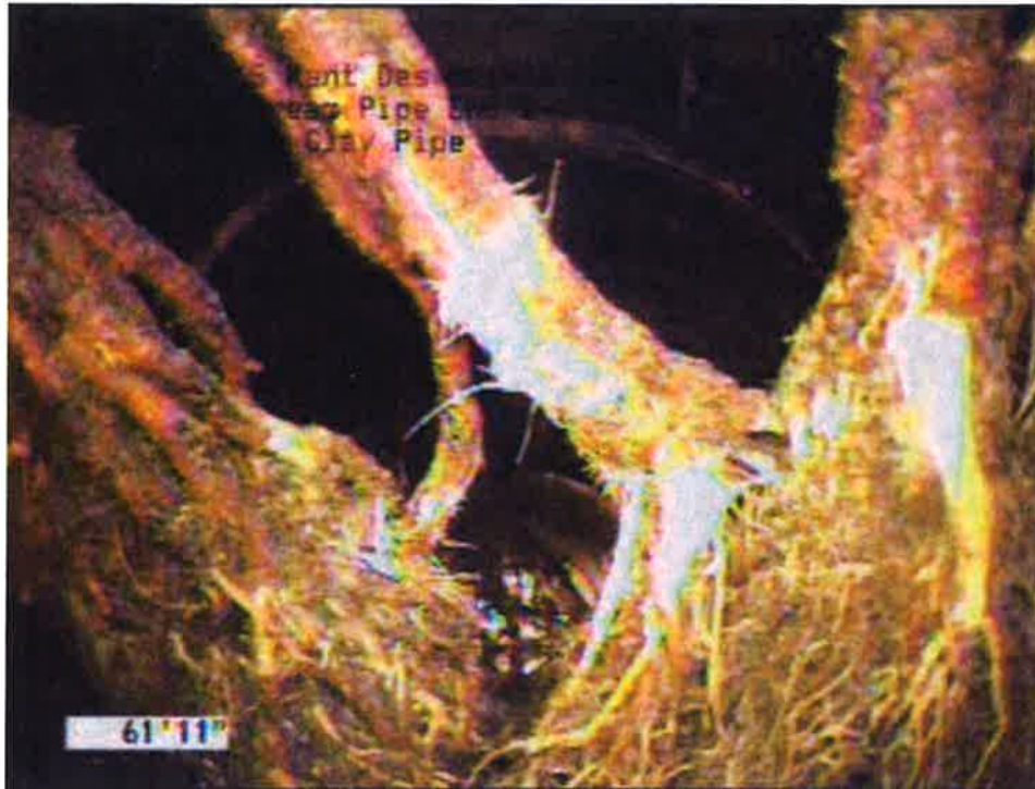
Photo 7 – Extensive Root Penetrations (outlet of culvert visible in the background)
