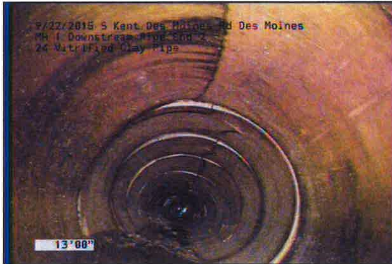
Photo: NA_MH 1_Pipe End 2_S Kent Des Moines Rd_22092015_130536_A.JPG, VCR No.: 9.22.2015 13.6FT, Fracture Longitudinal, at 11 o'clock, within 8 inches of joint: YES
