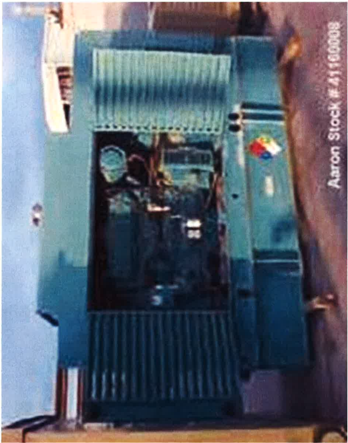
City Hall Generator
